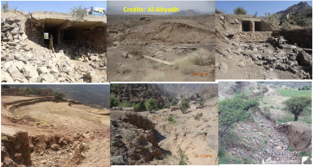
Photo 2.24 Erosion at culverts outlet due to the concentration of water
