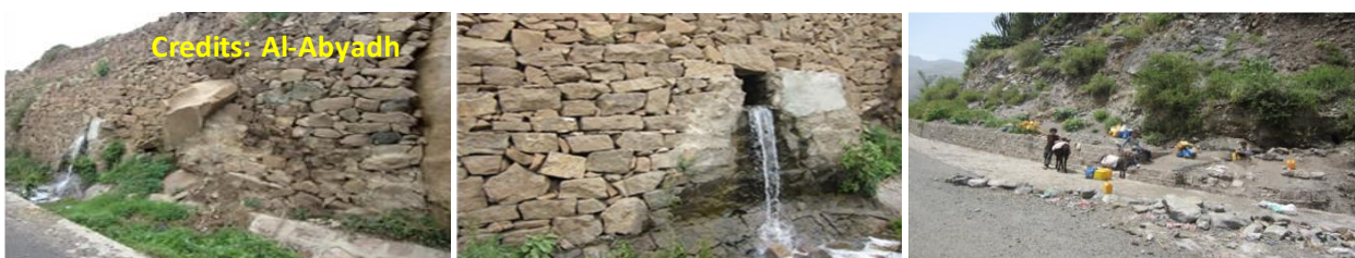
Photo 3.19 water spring water at uper slope of the road and drain to longtiudinal inside drain
