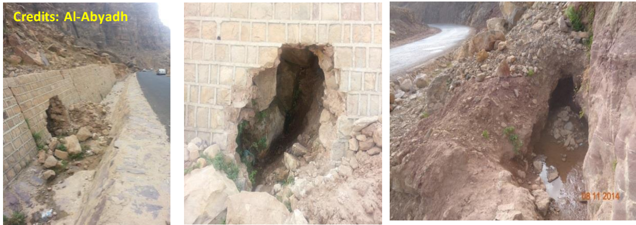
Photo 3.17 Pictures show neglecting the spring during road construction works in Yemen
