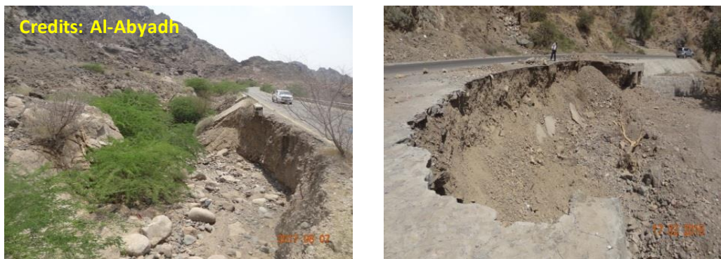
Photo 2.26 Erosion at road embankment due to concentrated of huge flood at the wadi beside the road ROW and due to the Prosopis Julifora (mesquite tree obstruction of the wadi flood waterway)
