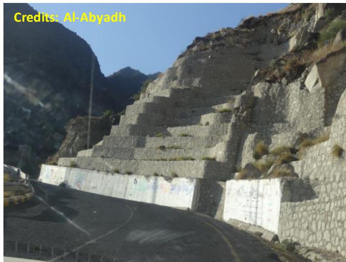
Photo 2.44 Example of Land Slide Protection Terraced Stone Masonry Walls at road cut side section
