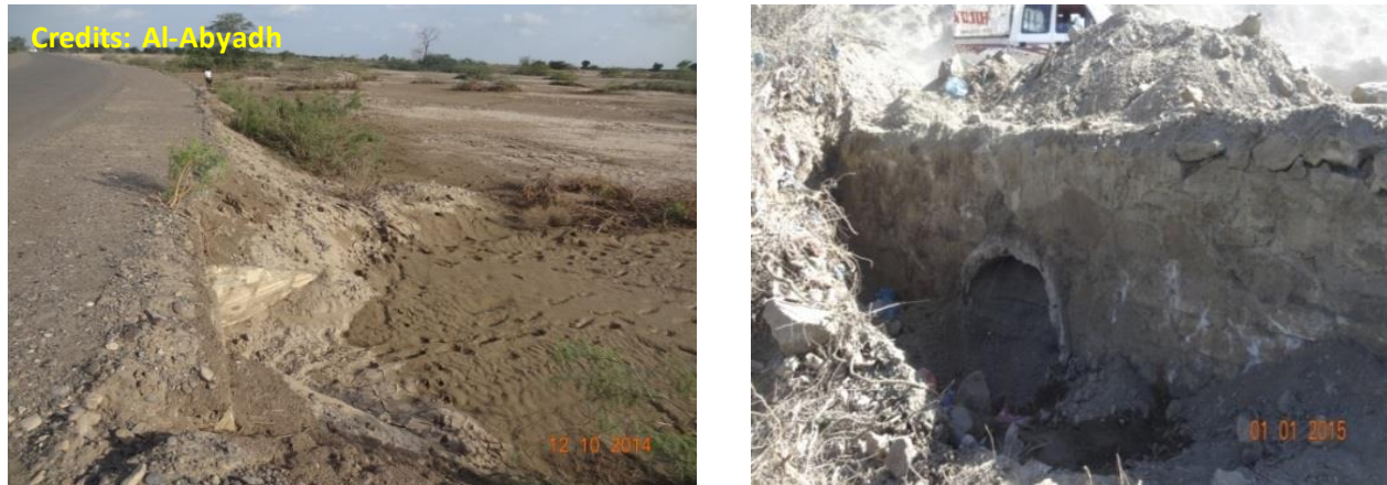
Photo 2.33 Sedimentation and siltation at culverts outlets/inlets
