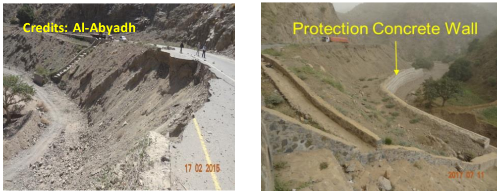
Photo 2.25 Erosion at road embankment due to concentrated huge flood at the wadi beside the road ROW
