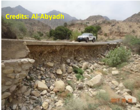
Photo 2.30 Scour at the Irish Crossing outlet due to the concentration of wadi flood water
