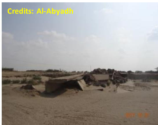
Photo 2.31 Scour and collapse of wadi Mawr Irish Crossing structure due to the huge seasonal floods
