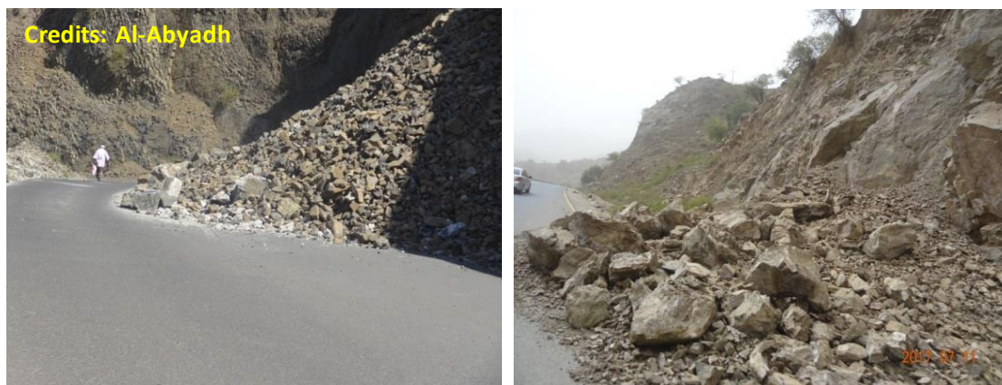
Photo 2.34 Land slide of loss rock cut causing disturbance and failure of retaining walls
