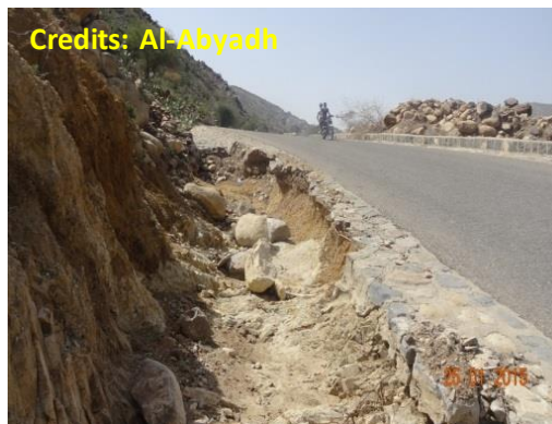
Photo 2.28 Erosion at road side drainage ditch and side protection works
