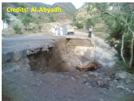
Photo 2.32 Scour and erosion at culvert outlet in wadi Lahima ( Al-Mahweet Gov.) box culvert structure due to the overload floods
